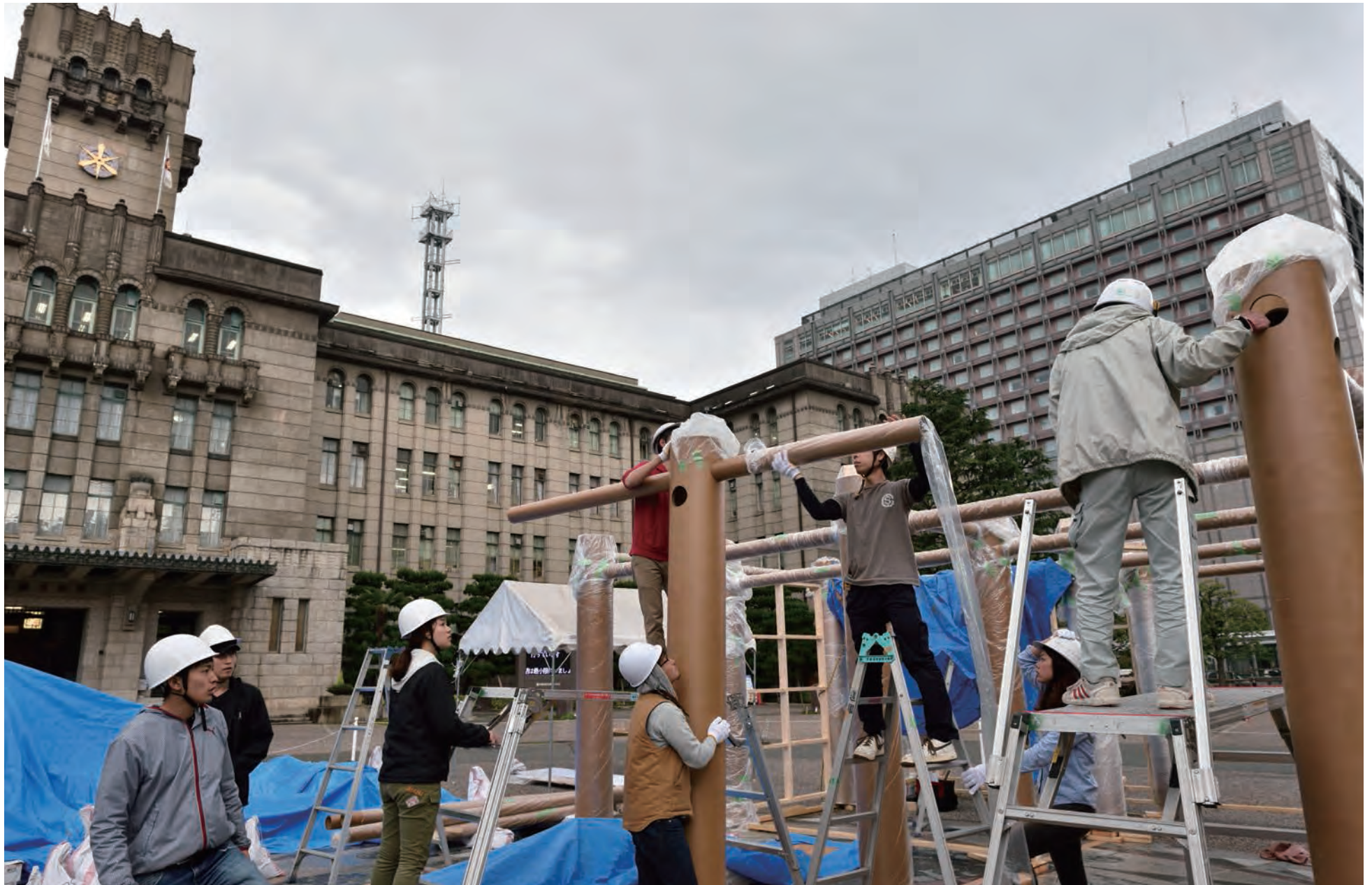
Students of Kyoto University of Art and Design constructing the Shigeru Ban Pavilion for the Martin Gusinde exhibition
